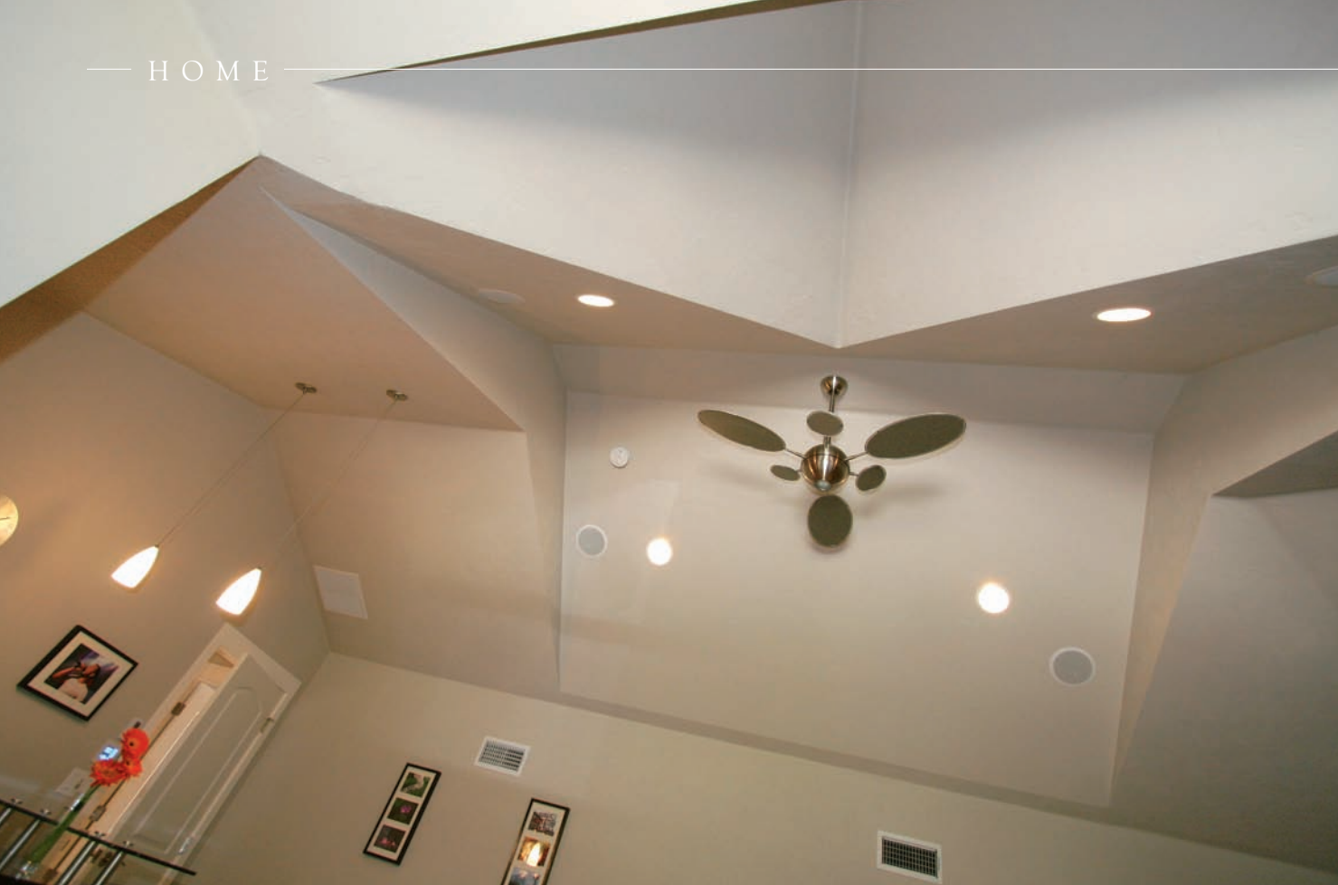
Above: Efficient yet abundant lighting illuminates the home. Left: Inset alcoves show off the family's art.
